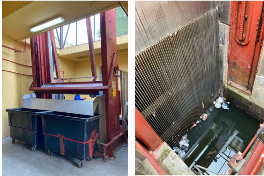
Figure 48: Example of one of the Pump Stations in the City of Miami
