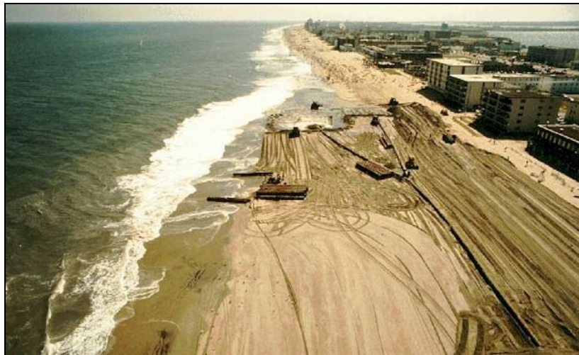
Beach renourishment project in Ocean City (photo: Rutgers University, Institute of Marine and Coastal Sciences, http://marine.rutgers.edu/qgeomorph/oceancityfill.jpg ).
